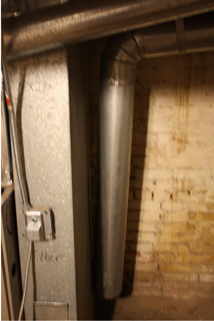
Hot Water Heater:
